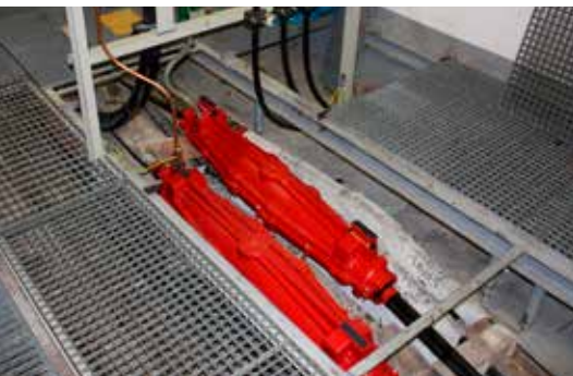
Olienavulmoffen in schakelstation
