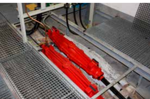
Olienavulmoffen in schakelstation
